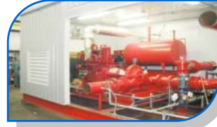
Fire Protection System Audit Report (Form - B)
