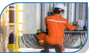
Electrical Safety Audit
